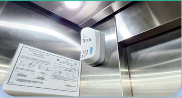
Installation of 126 Units Room Scenting Devices January 1, 2025
