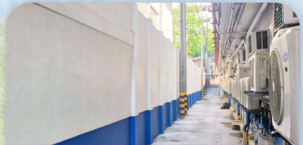
Reconstruction and Retrofitting of Eusebio Wall and Exit Driveway Wall Between Immaculate Heart of Mary College October 24, 2024
