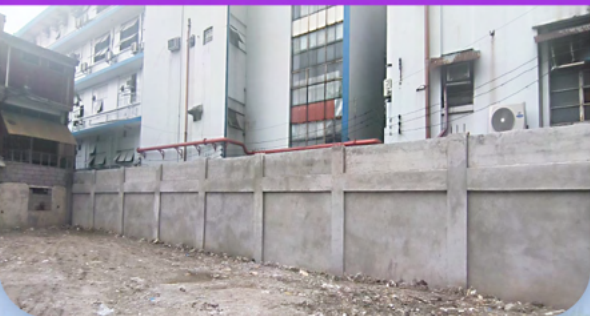
Supply and Install of CHB Wall and Gate at Eusebio Compound September 30, 2024
